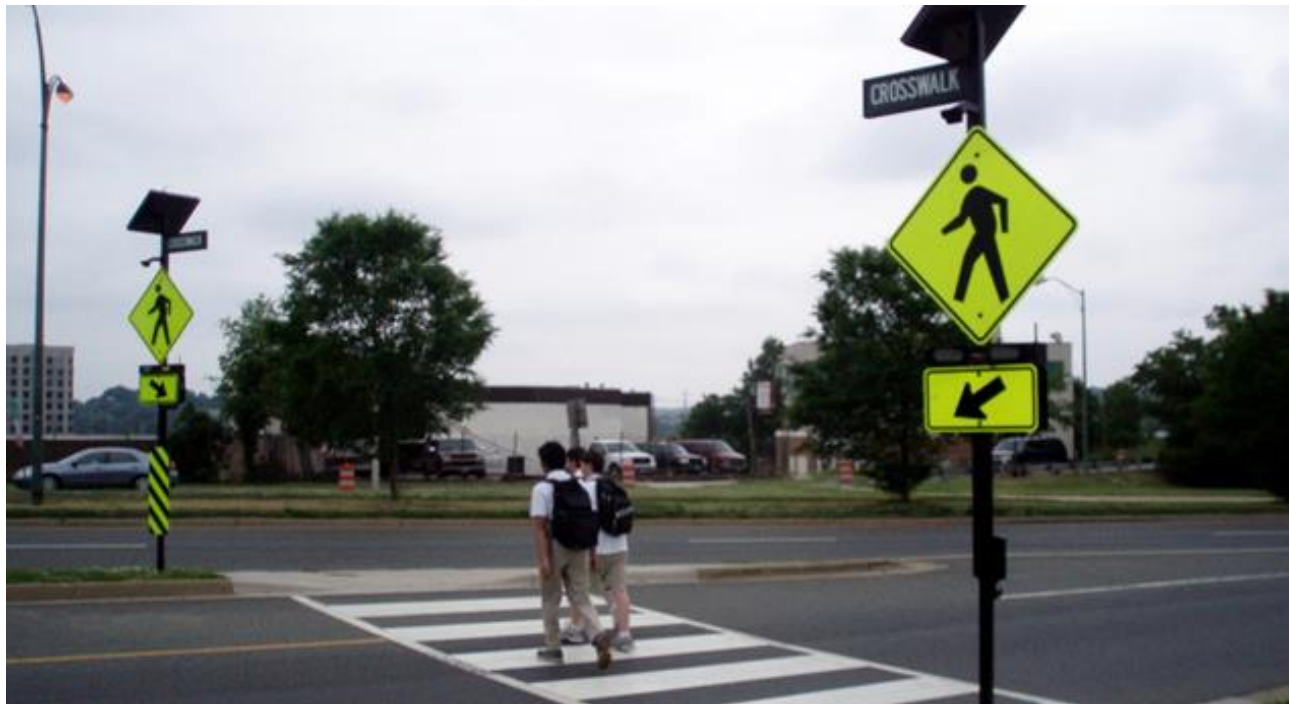
Figure 25: Rectangular Rapid Flash Beacons (RRFBs)
