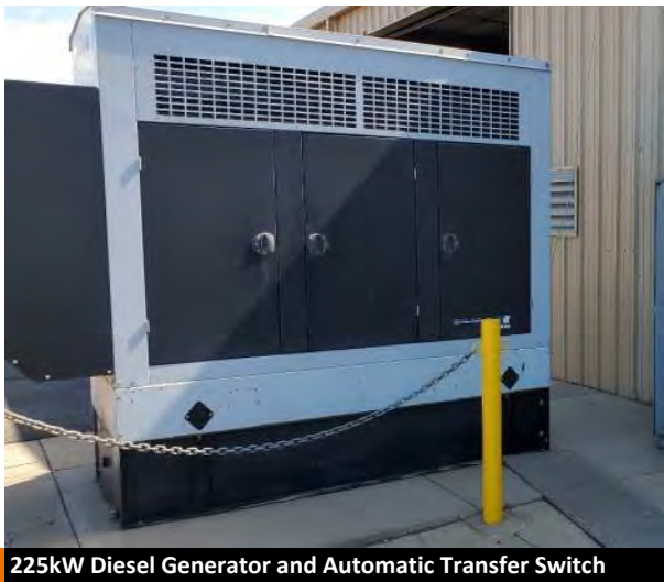
G5.1 225kW Diesel Generator and Automatic Transfer Switch
