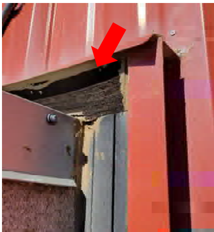
D1.3 Horizontal Expansion Joint Cover - Aging
