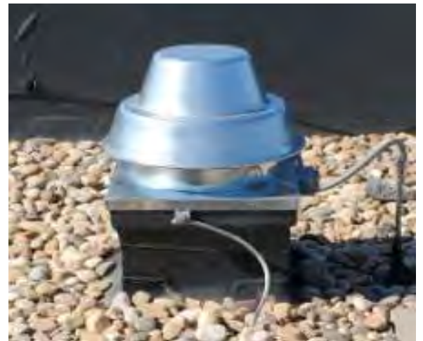
F12.1 Roof mounted exhaust fan.
