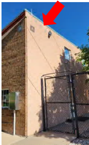
B3.1 Stucco Veneer - Wood Pecker Holes
