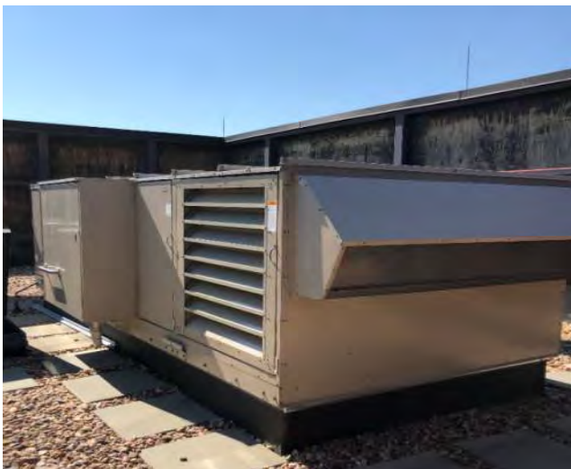
F11.1 Rooftop unit outside air intake.
