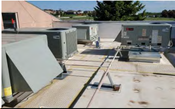
F11.1 Typical outside air intake on rooftop units.
