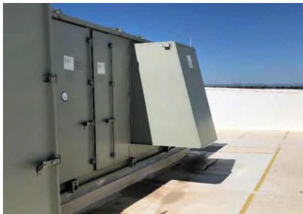
F11.1 Outside air intake on rooftop units.
