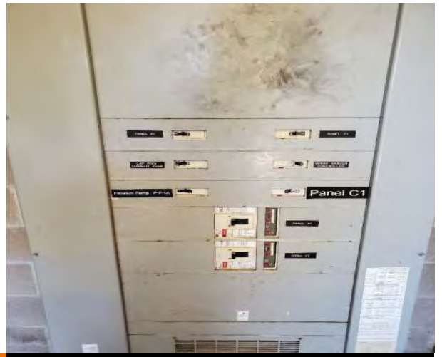
G9.1 Main Switchboard with Surface Rust
