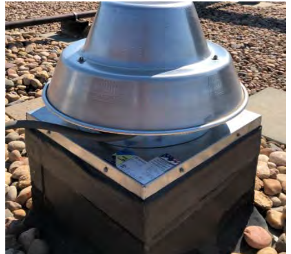
F12.1 Roof mounted exhaust fan.
