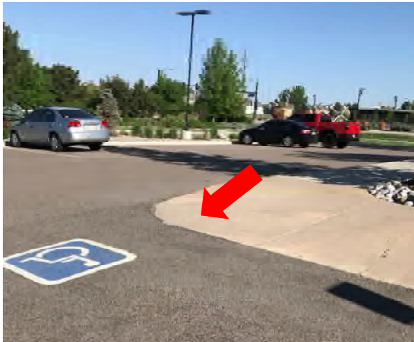
B2.1 Full curb recommended to emphasize ped vs vehicular areas (this is not an acceptable ADA ramp)
