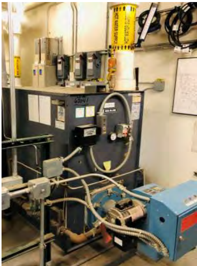
F9.1 Boiler for heating water.
