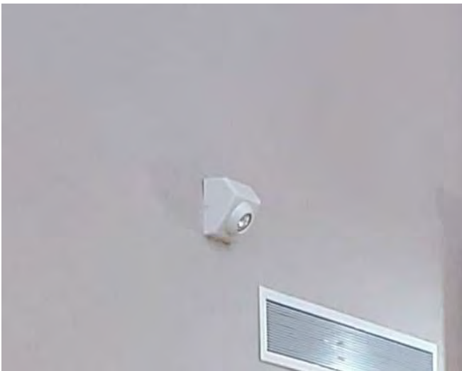
G4.1 Main Entrance LED Egress Fixture
