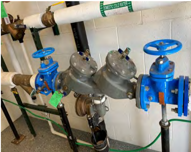
F1.1 Domestic Water Entry
