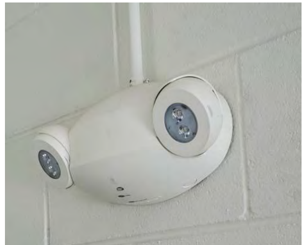
G6.1 Typical Battery Backed-up Dual Lamp Egress Fixture
