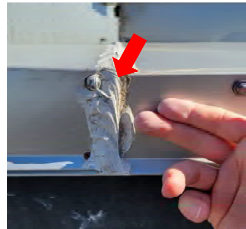
D1.4 Flashing Joint Caulking - Aging
