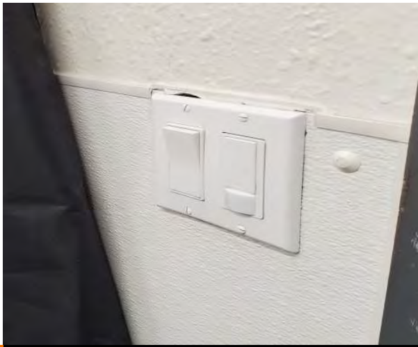
G1.1 Combination Toggle and Occupancy Sensor
