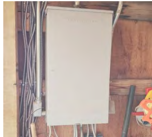
G8.1 150A Panel In Nema 3R Enclosure
