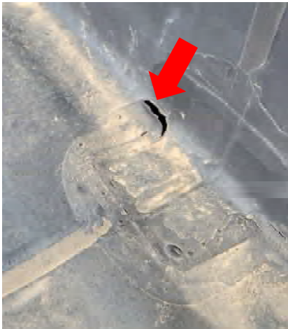
D1.1 Black EPDM Roofing - Failing Joint
