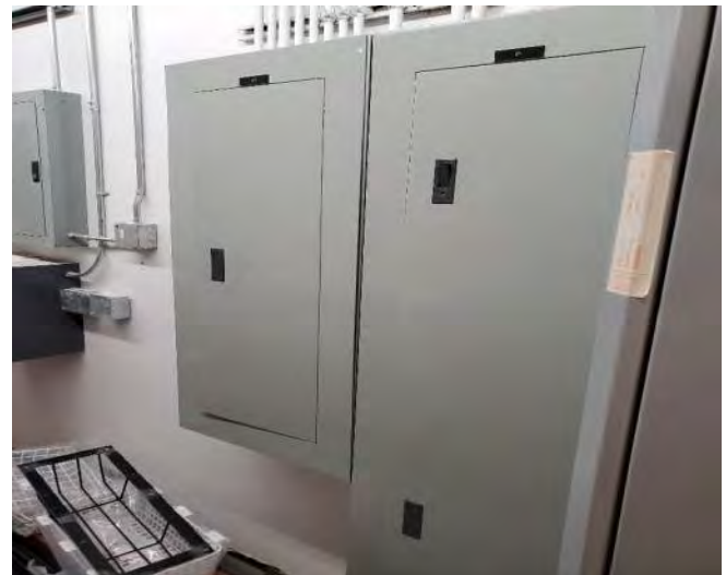
G8.1 Branch Distribution Panels
