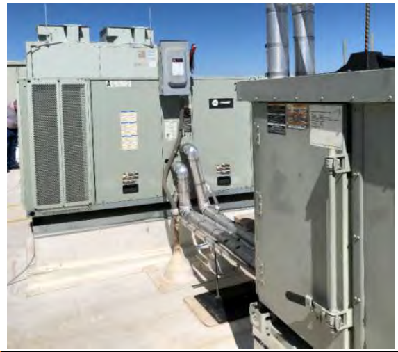
F10.1 Typical rooftop condensing unit.
