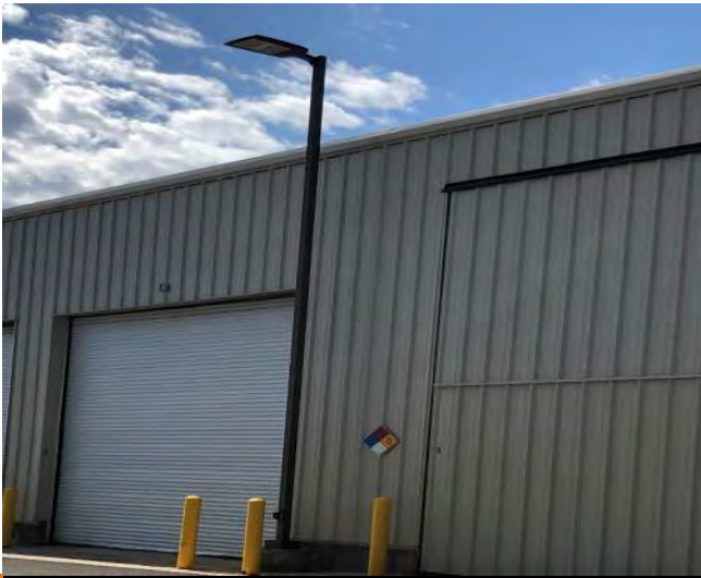
G2.2 Exterior Pole Mounted LED Fixtures
