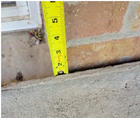
D5.1 Concrete Floor - Heave / Settle
