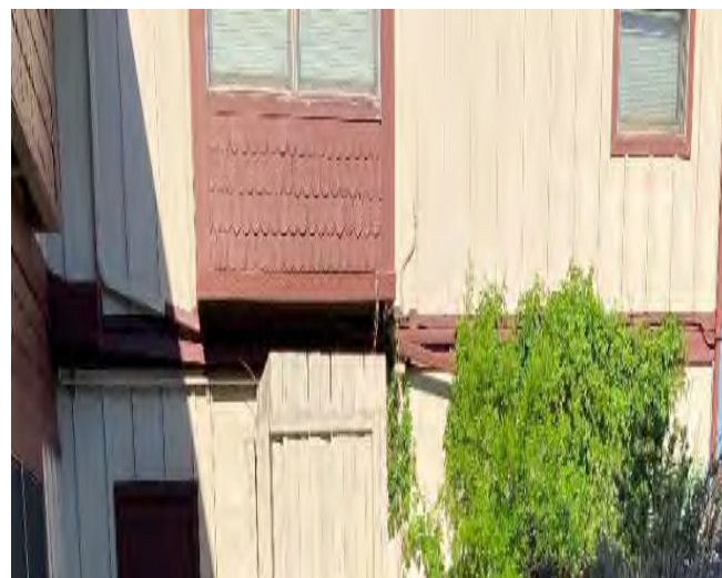
F4.1 Rain Gutters and Downspouts Leak
