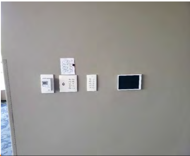
G1.1 Programmable Lighting Control Station
