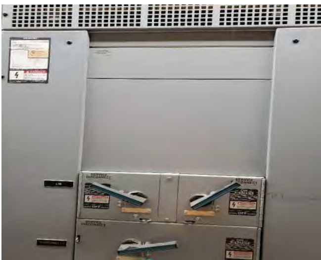
G9.1 1200A 277/480V Main Distribution Panel
