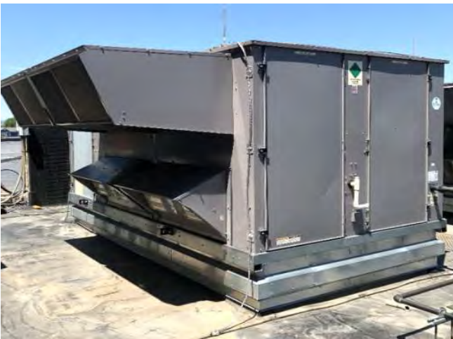
F11.1 Typical outside air intake and power exhaust on rooftop units
