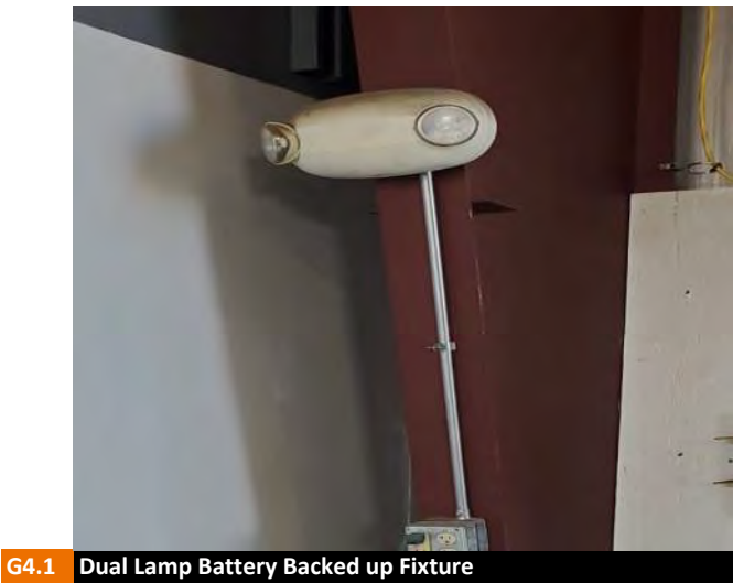
G4.1 Dual Lamp Battery Backed up Fixture
