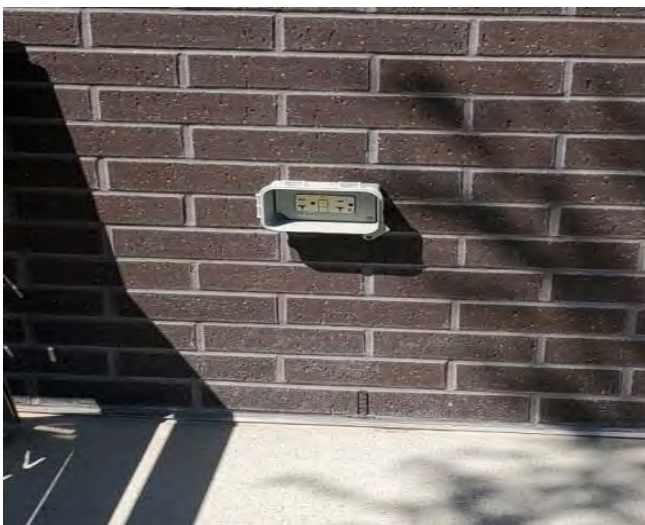
G10.1 Exterior Weather Proof Receptacle Missing "In-Use" Cover
