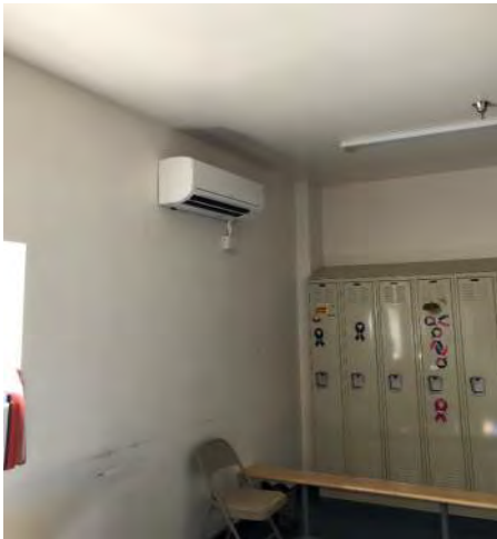
F11.1 Outside air not provided to locker room or break room.
