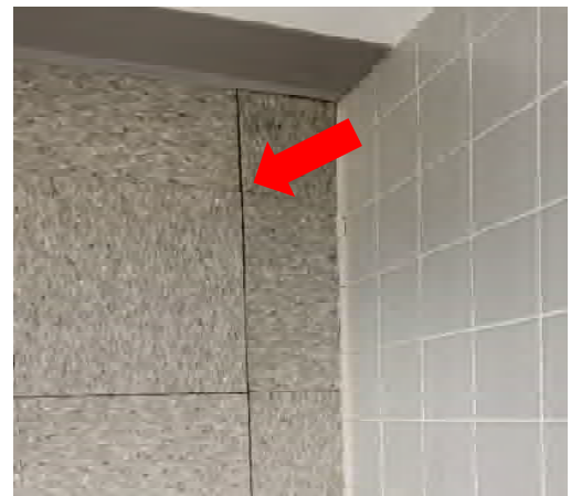
D6.1 VCT Tile - Gaps
