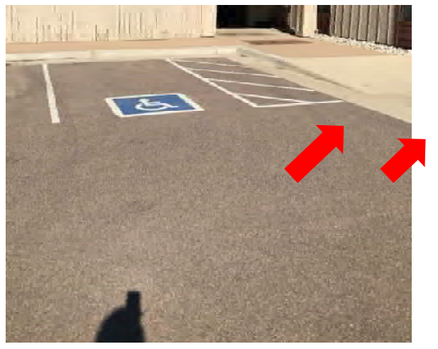
B7.1 East ADA space requires extension of striping to ramp, and truncated domes on ramp
