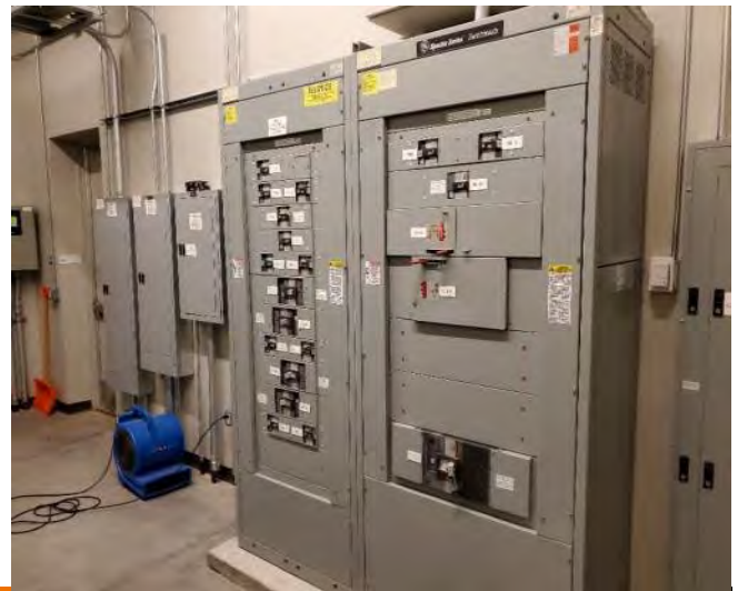
G9.1 1600A 277/480V Main Distribution Panel
