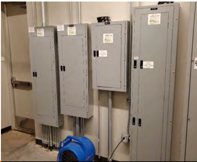
G8.1 Branch Distribution Panels
