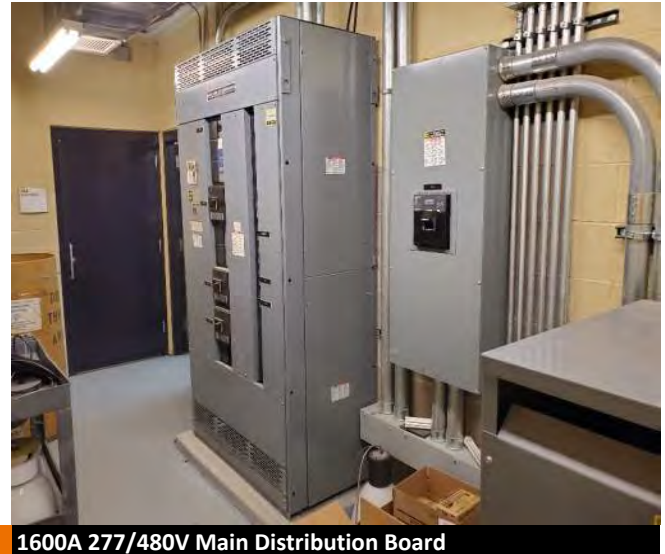
1600A 277/480V Main Distribution Board
