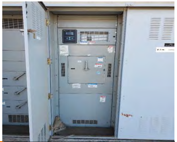
G9.1 800A Main Distribution Switchboard, NEMA 3R Enclosure
