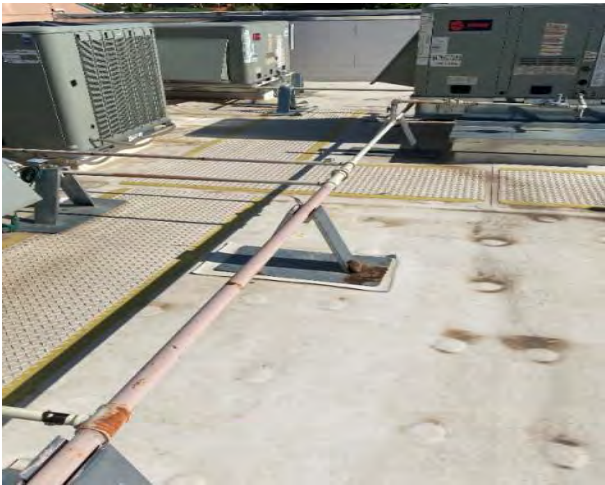
F2.1 Natural Gas Piping Serving RTU
