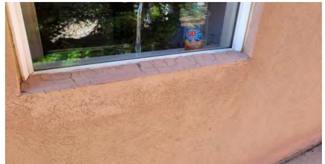
B4.1 Stucco Sill - Cracking
