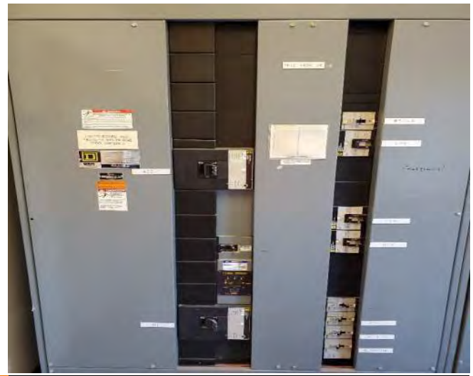
G9.1 1200A 277/480V Main Switchgear
