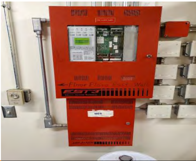
G6.1 Addressable Fire Alarm Control Panel
