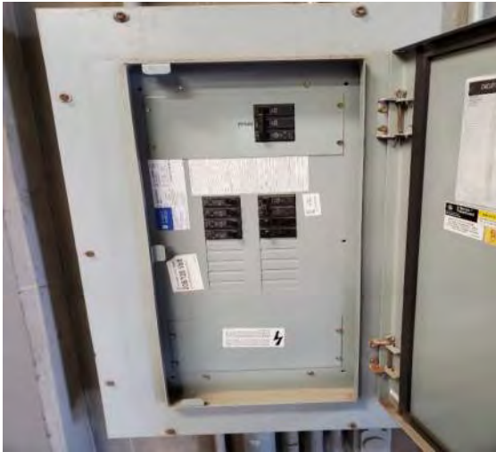
G8.1 120/208V Panelboard With 60A Main Breaker
