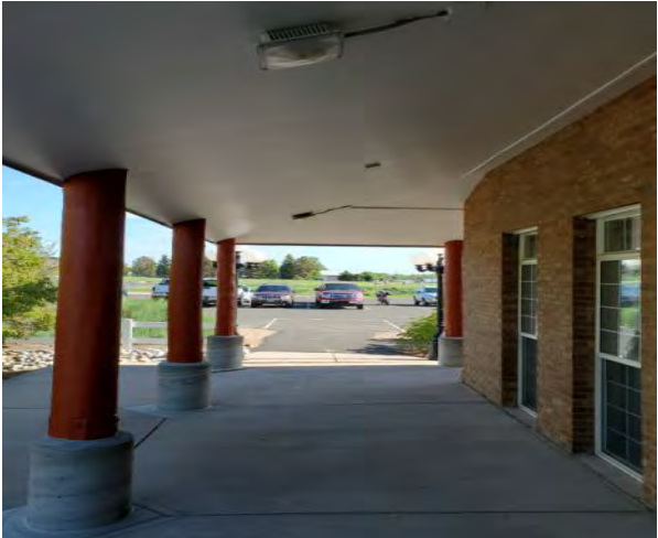
F4.1 Pitched Roof Area With No Gutters
