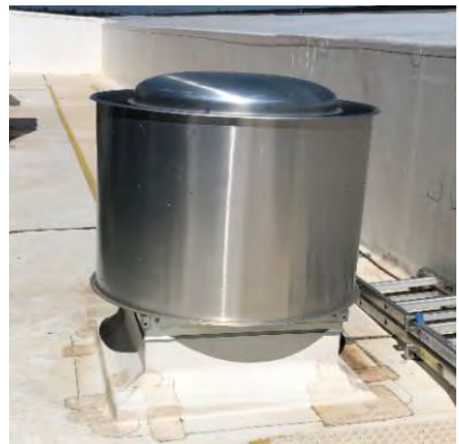
F12.1 Roof mounted exhaust fan.
