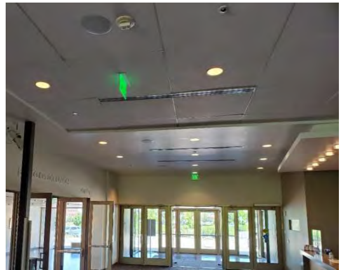
G2.1 Main Entrance Downlights and Decorative Fixtures
