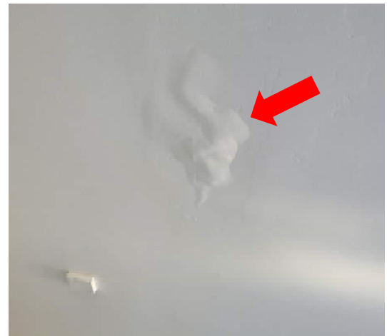
D4.1 Gypsum Board Soffit/Ceiling - Bubble
