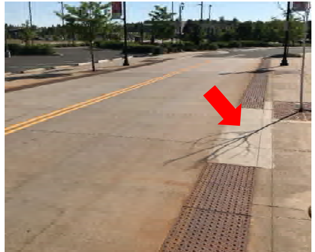
B3.1 Missing section of truncated domes along entry
