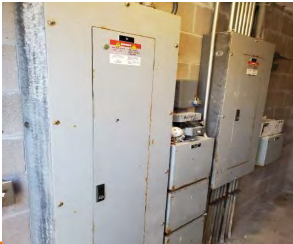
G8.1 Branch Distribution Panels with Surface Rust
