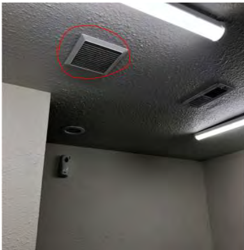
F12.1 Typical ceiling exhaust fan.
