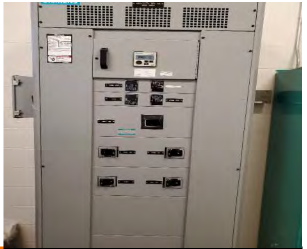
G9.1 1200A 277/480V Main Switchgear
