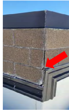
D1.2 Effervescence at Pool Wall Parapet
