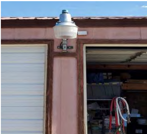
G3.1 "Goose Neck" Fixtute wit LED Retrofit Lamp
