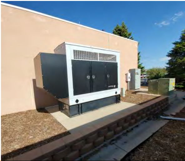
F7.1 Emergency Generator Conflict With Sewer
