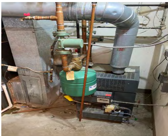
F1.1 Snow Melt Boiler
