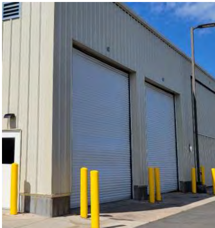
D2.2 Overhead Coiling Doors
