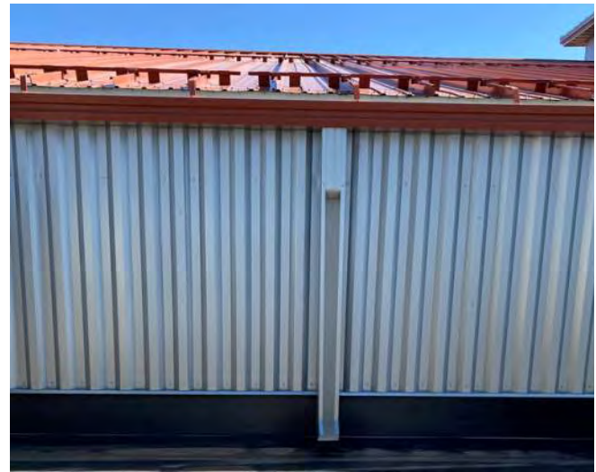
F4.1 Rain gutter and Downspout
