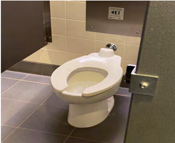
F3.1 Plumbing Fixtures Have Electronic Control
