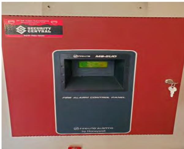
G6.1 Addressable Fire Alarm Control Panel
