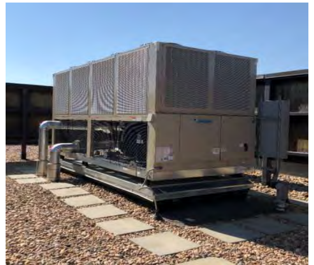
F10.1 Daikin chiller.
