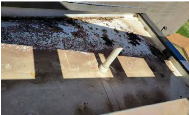
D1.5 Debris on Roof
