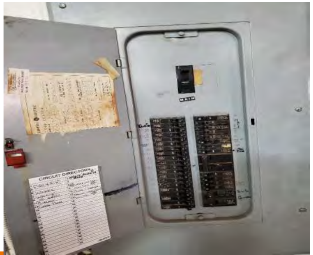
G8.1 200A Main Distribution Panel
