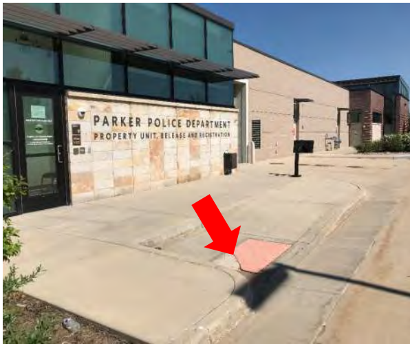
B4.1. Damaged truncated domes at east entry
