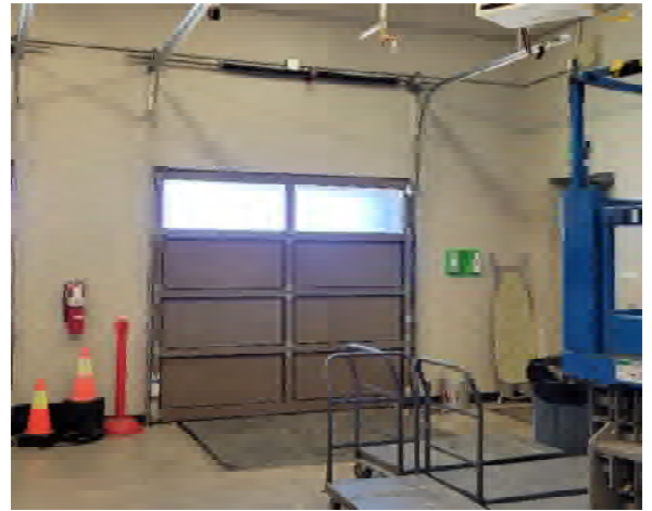
D2.3 Overhead Doors
