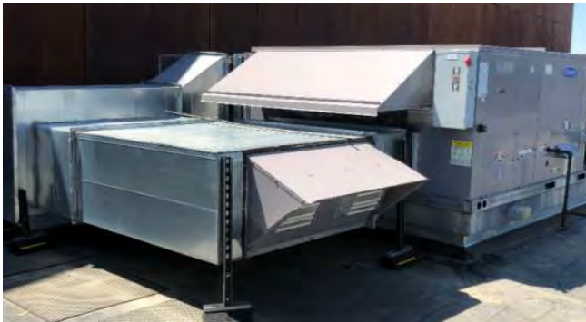
F9.1 Typical gas-fired heating rooftop unit.
