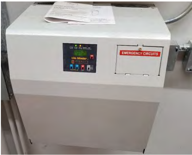
G5.1 Court Lighting Battery Inverter
