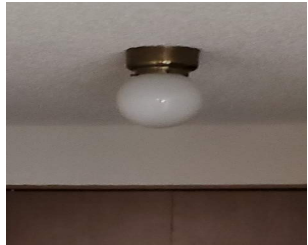
G2.1 Incandescent Fixture in Hallway
