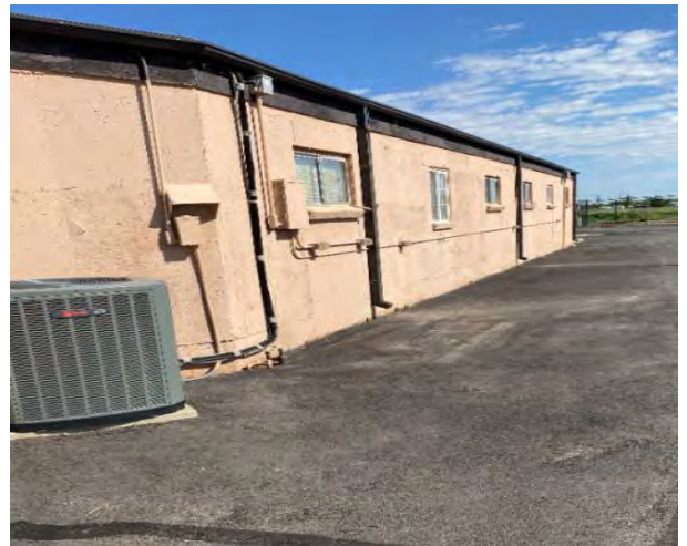
F4.1 Partial Rain Gutters. Not installed All Around
