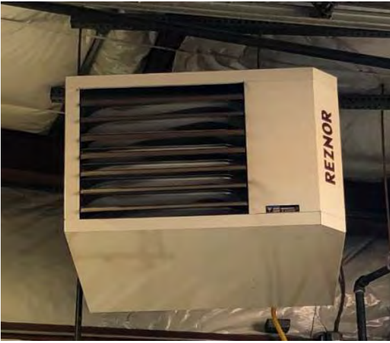
F9.1 Typical gas-fired unit heater.
