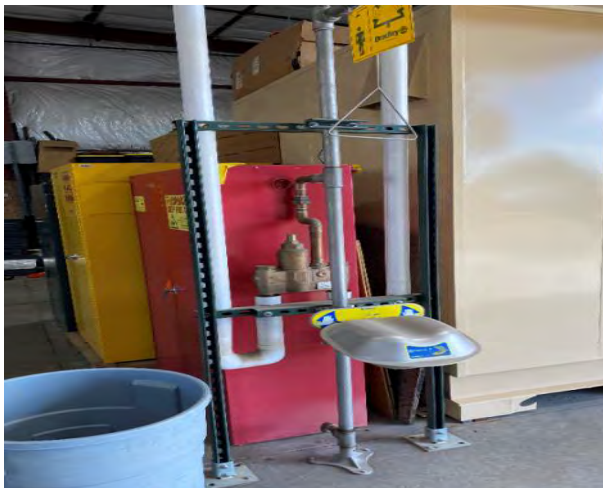
F6.1 No Tempered Water On Eye Wash
