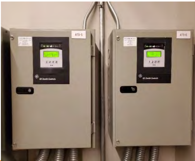
G5.1 Life Safety and Stand-by Automatic Transfer Switches
