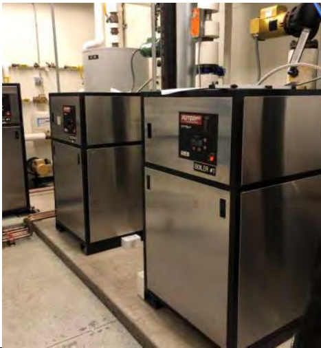
F9.1 Heating water boilers.
