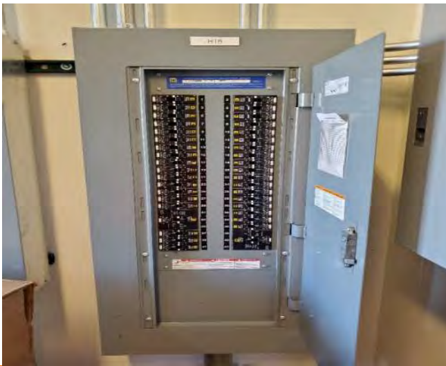
G8.1 Typical Square D Panelboard
