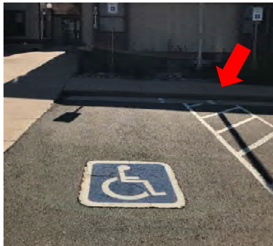
B7.1 West ADA spaces do not meet dimensional standards; require wheel stops and ramp with truncated domes in access aisle
