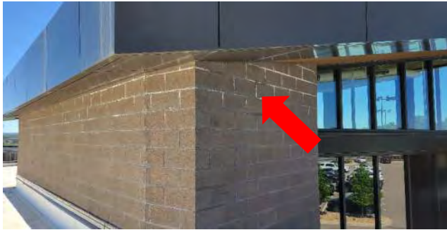
D1.1 Effervescence at Water Slide Tower
