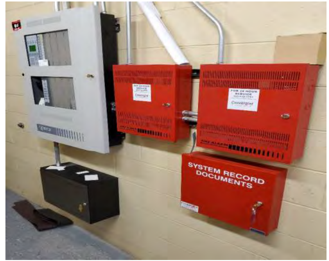
G6.1 Addressable Fire Alarm Control Panel
