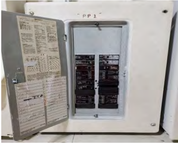
G8.1 Typical ITE Panelboard
