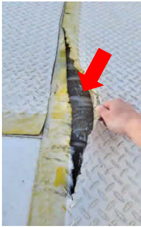
D1.7 Walkway Pad - Damaged
