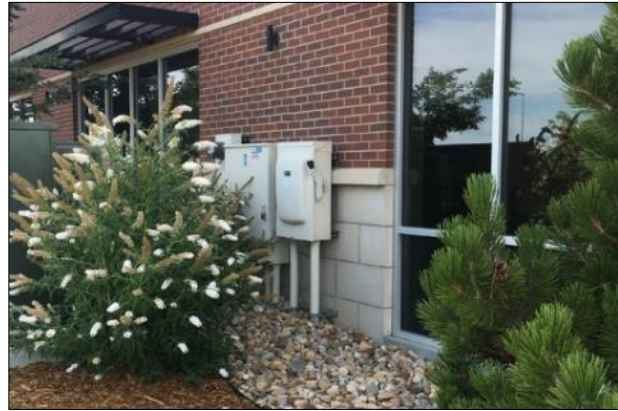
Figure 63 - Landscape-screened utility boxes attached to a building.
