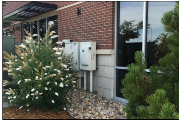
Figure 63 - Landscape-screened utility boxes attached to a building.
